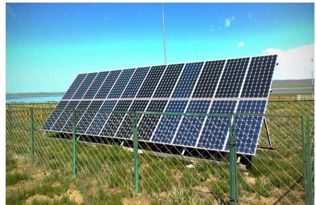
Fig.1. An Installation of 24 solar modules in rural Mongolia
